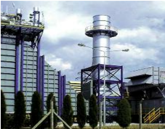
Picture above: view of the combined cycle power station Entek , Turkey with the bypass system in the centre.
