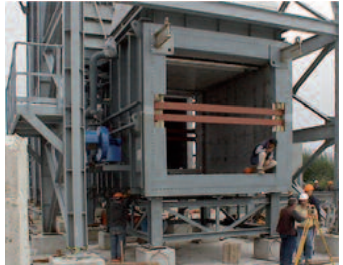
Diverter with bypass system during erection at Ostim power station in Turkey with a RAUMAG-JANICH supervisor in attendance
